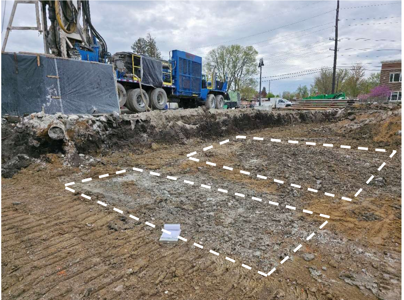
Photo 3. Approx. Extents Soft Wet Clays near Eastern Wall, Looking Southeast
